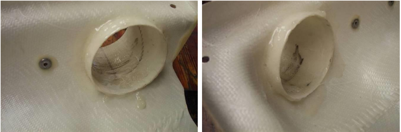
Figure 34. Air Filter Box Plumbing – Incorrect
